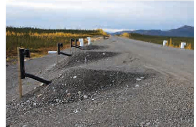
3.33 > Roads built on permafrost generally subside first at their verges, where the frozen subsoil thaws fastest. Thermosiphons are installed to prevent this happening. They convey ice-cold air in winter to the still relatively warm subsoil, thus keeping it cooled.
