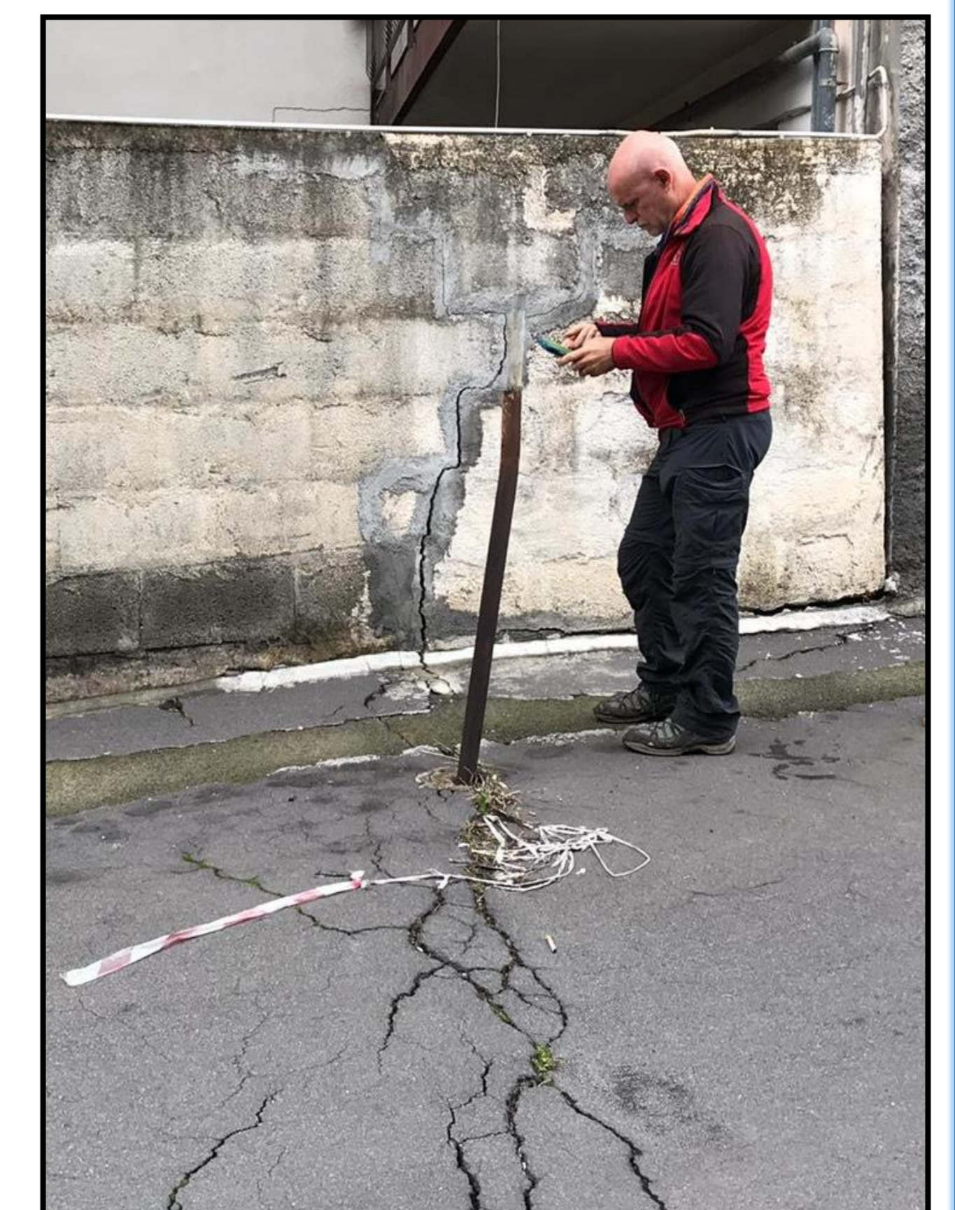
Fig. 3: Ruptures on the ground and a wall along the Aci Catena Fault.
