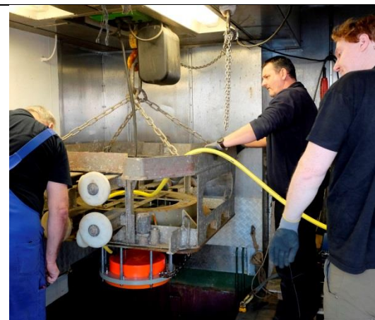
Figure 1: Installation of the 38 kHz transducer (EK80, red instrument) at the moonpool (from left to right: Peter Neumann, Olaf Willms, Florian Gausepohl). [Photo credit: Peter Urban]
