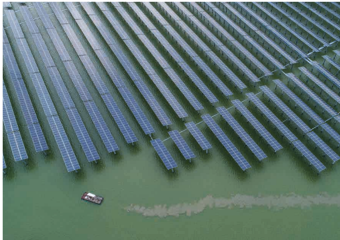
5.33 > Photovoltaic arrays so far have been primarily located in shallow bays where they are protected from wind and waves. This installation in the Chinese coastal city of Zhangzhou is one example.
