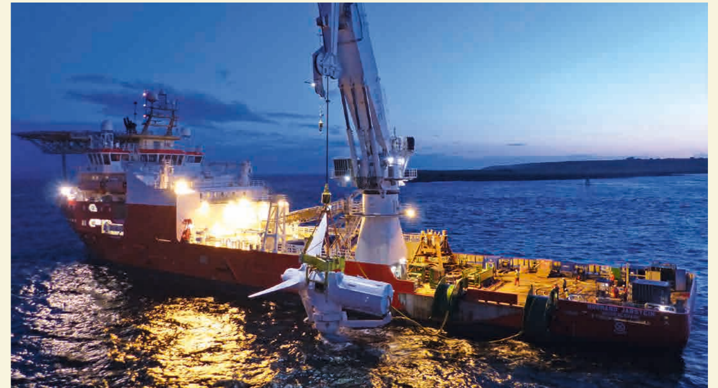
5.32 > One of the fastest marine currents of Scotland drives the underwater rotors of the MeyGen power plant. In the first phase, the operating company installed four turbines on the sea floor, which have been supplying around 2600 households with electricity since August 2018. Further turbines will be added.
